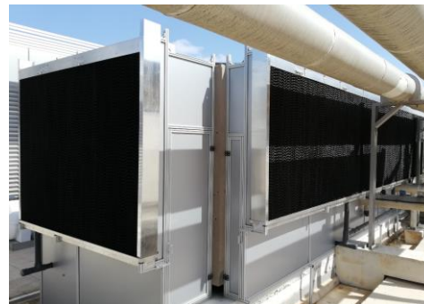
Chiller Evaporative Cooling Membrane
