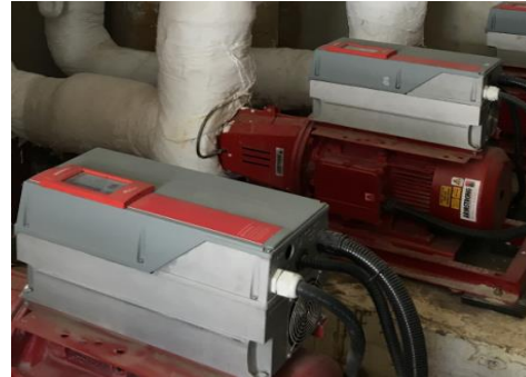
New VFD controlled chilled water pumps
